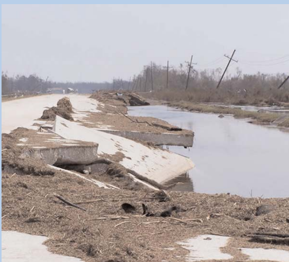
A Louisiana highway succumbs to the force of Hurricane Katrina.
