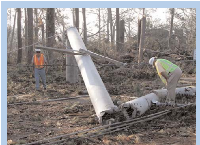
Utility crews examine a snapped pole during last year's hurricane season.
