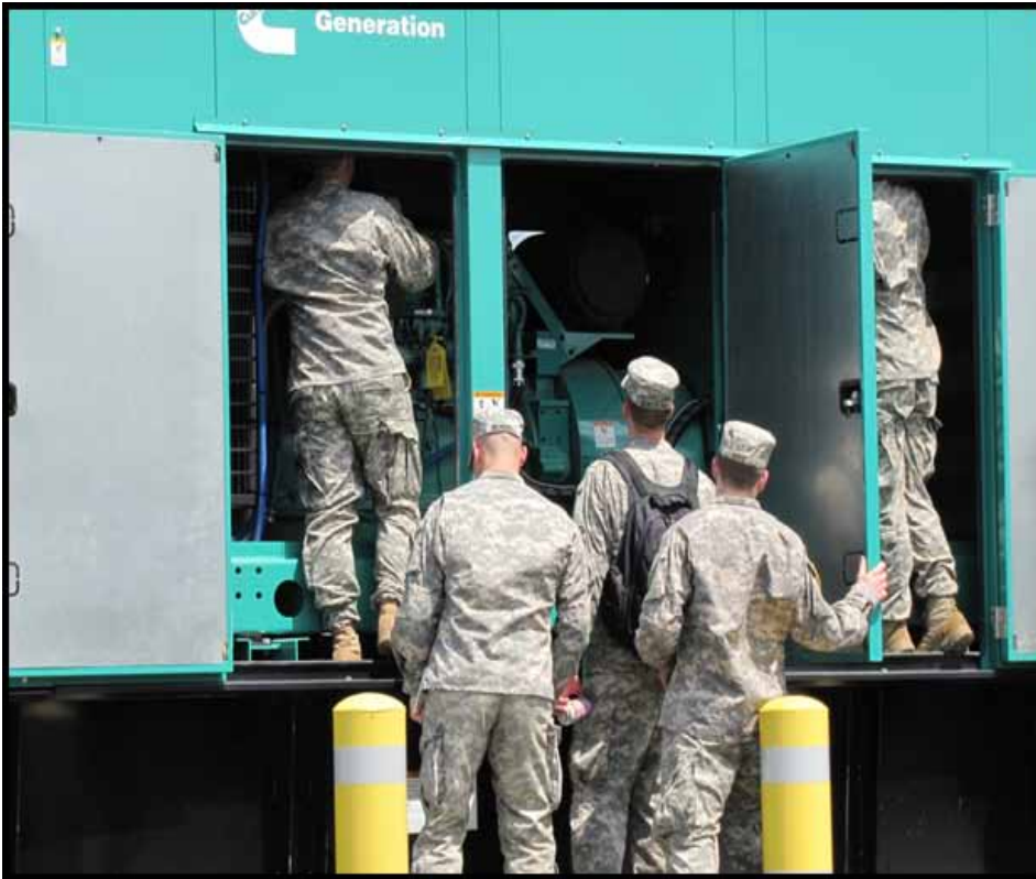
Figure 4: Cadets inspect an emergency backup generator at the West Point Transportation Motor Pool. Photo by Led Klosky.
