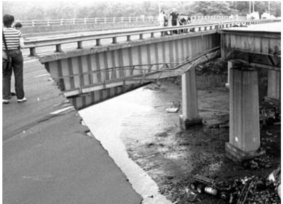
Figure 1. The Mianus River Bridge Following Collapse of the Northbound Span in 1983
