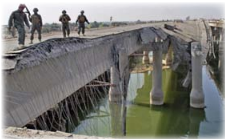
Figure 1: Vehicle Borne Improvised Explosive Device (VBIED) Damage to Bridge in Iraq (2009).
